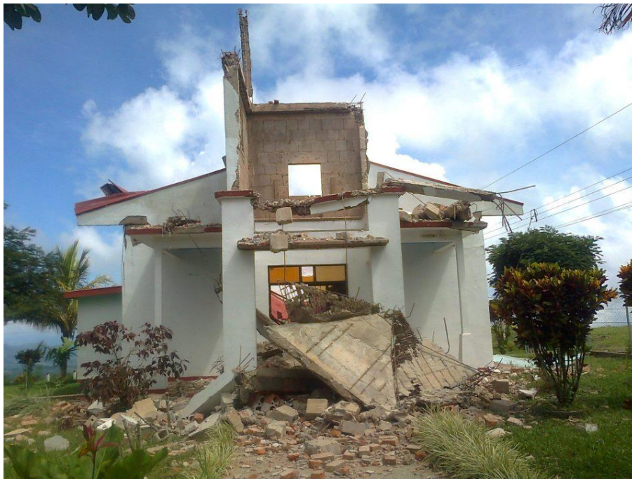
Damaged church in Buena Vista in Nandayure (Guanacaste province)
