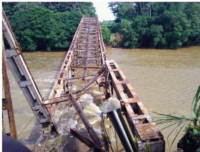
Bridge collapsed on Rio Sucio
